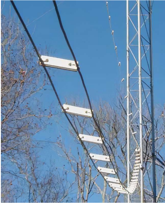
Figure 1: Open Wire transmission line
